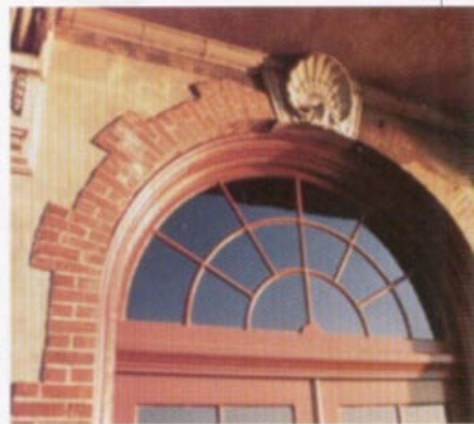
The landmark building's structure was predominantly sound, but its stucco and brick walls were beginning to show their age.
